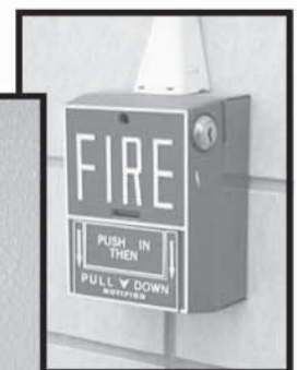
Fire Alarm Pull Station
